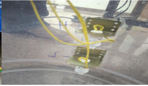
Figure 4: Level sensor inside tank
